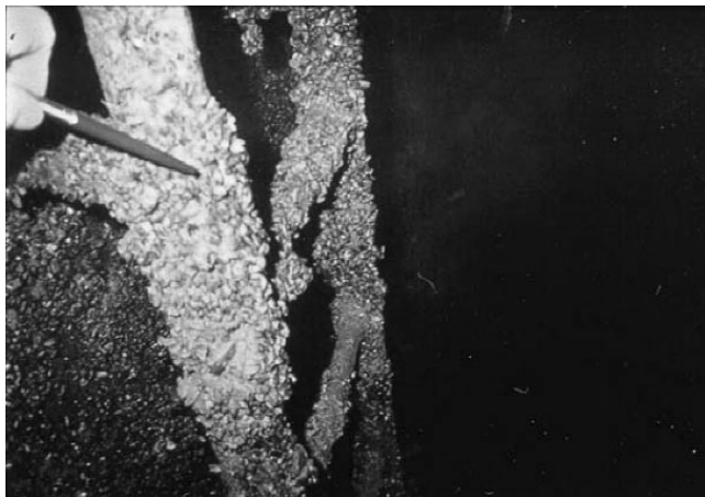
Figure 5: Zebra mussels colonizing a ladder in an intake structure.
