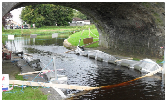
Figure 2. Impermeable curtains used to hold treated water within treatment area along canal walls. Photograph by Sara Meehan.
